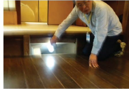
figure 28.13 Cool-tube outlet under the tatami room
