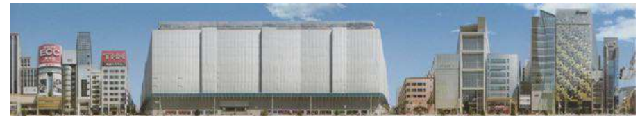
Figure 1: Street view of Chuo Dori with Ginza Six under construction (picture courtesy of Asahi Building Wall company). Although the 115-meter street frontage is out of context, the height of the complex was kept at 56 meters to fit into the street scape of the Ginza district.
