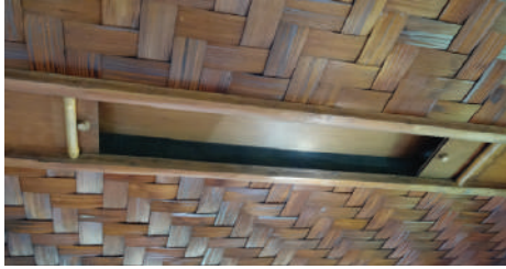
figure 28.11 Operable ventilation outlet on the ceiling of the engawa
