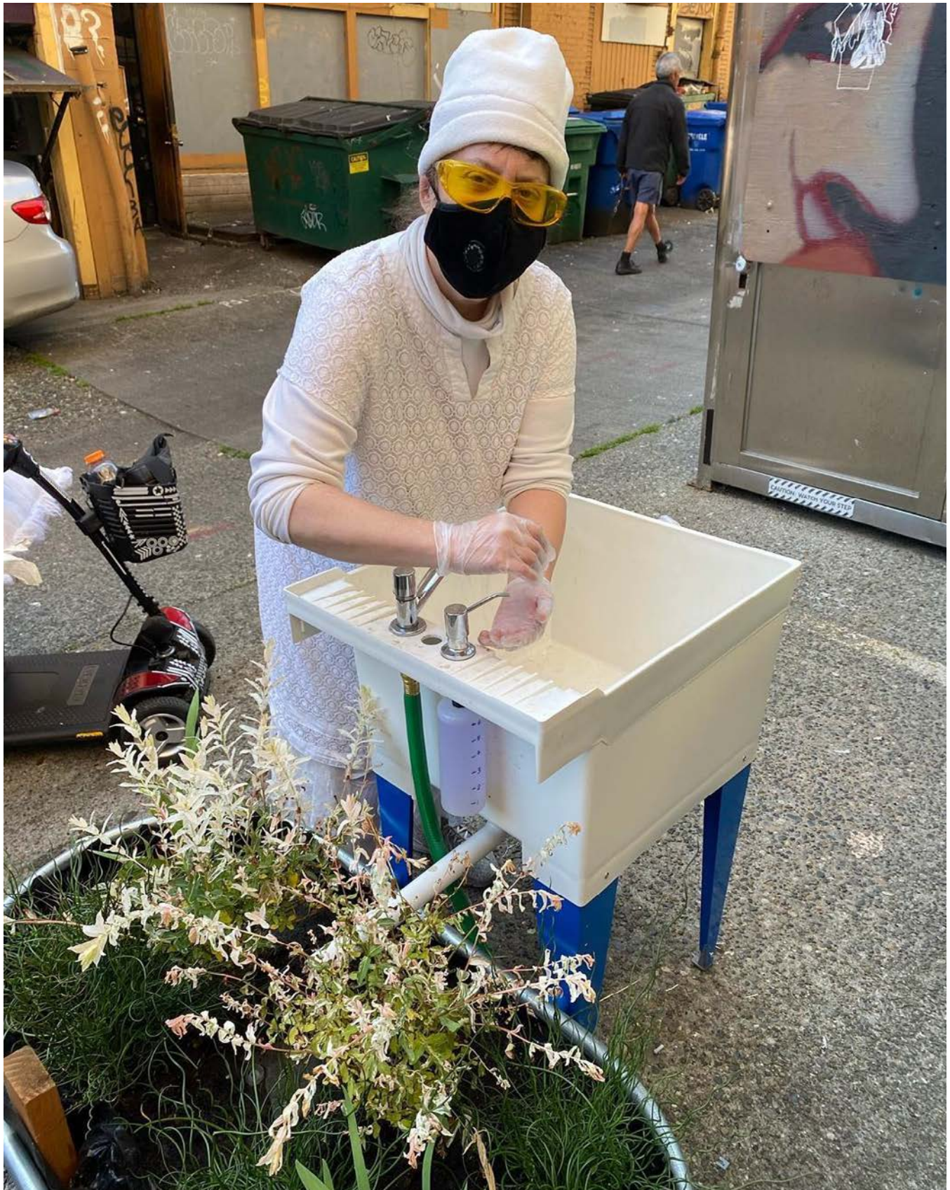
Figure 5. Seattle Street Sink located in alley behind ROOTS Young Adult Shelter. Brice Maryman.
