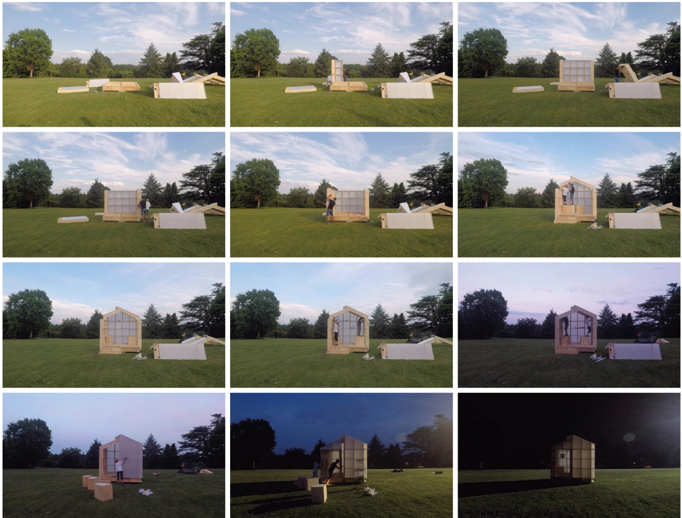
Figure 6. The process of disassembling and reassembling the structure for installation reinforced students' conceptual understanding of the project's fabrication and construction logics.
